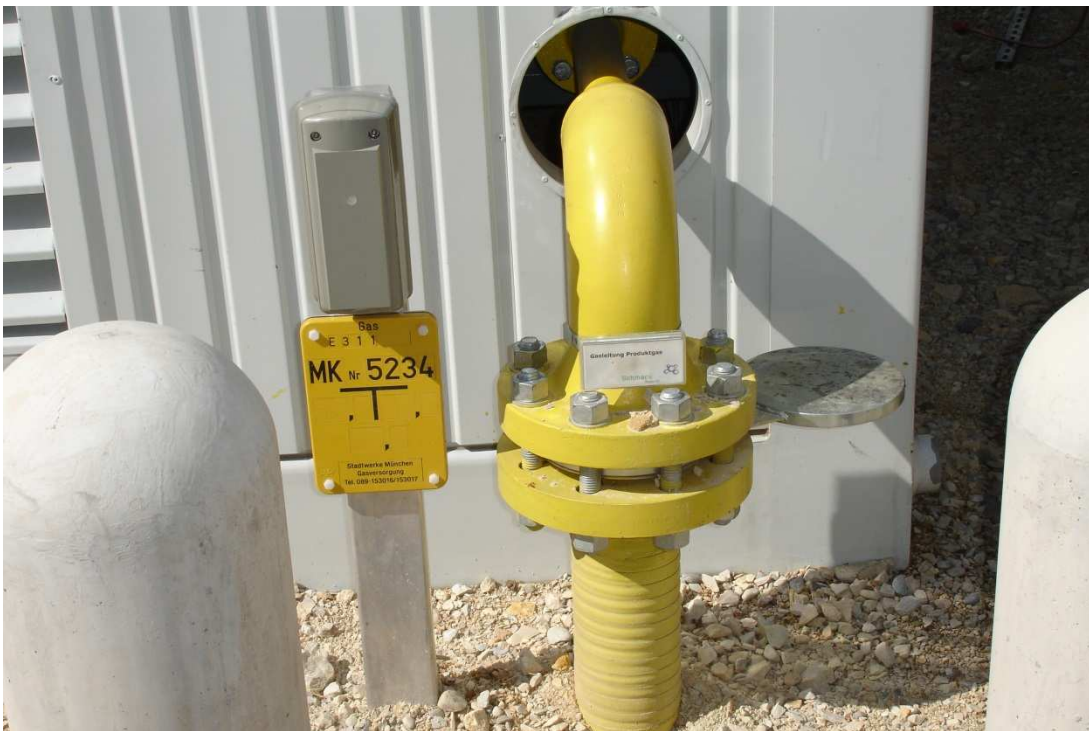
Figure 6.10: Treated Biogas leaving the plant for injection at Pliening Biogas plant near Munich
