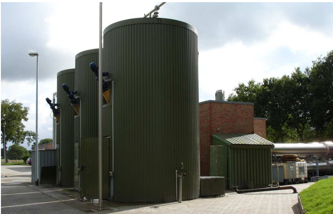
Figure 6.2 Fermenters in a biogas plant
