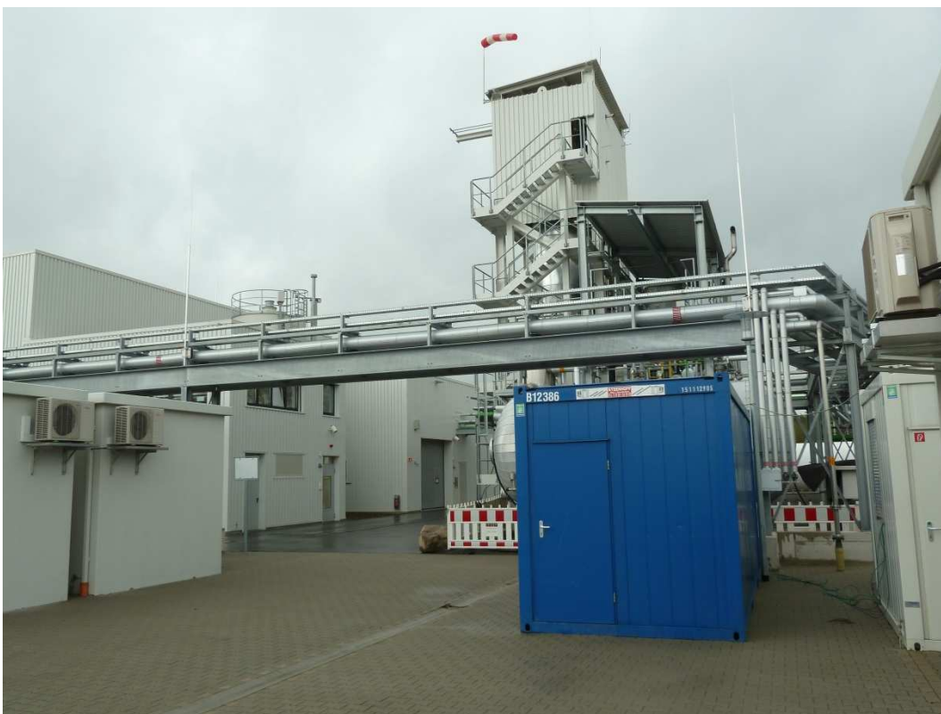
Figure 6.5: Partial view of the Audi™ methanation plant in Werlte
