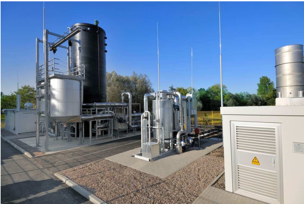
Figure 6.10: biomethane production and injection plant in Horn-Bad Meinberg, Germany
